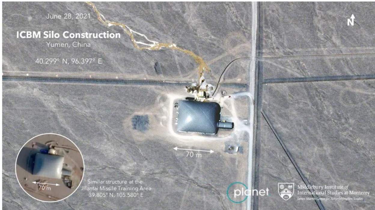
A commercial satellite photo taken Monday over northwestern China shows what experts say is a construction site for a new silo for a nuclear-tipped ICBM. The construction site is hidden under a 230-foot
