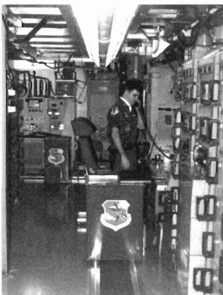
Interior of Launch Control Center (acoustical enclosure) showing the command and status consoles.
