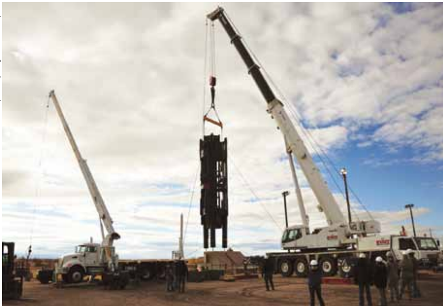
Left: A 47,000-pound missile support system is hoisted out of a launch training facility at Warren. While it's being repaired and refurbished, maintainers will perform corrosion control and other preventive maintenance in the silo. Below: An inert Minuteman III ICBM is lofted into space from Vandenberg AFB, Calif. Minuteman missiles are being upgraded and modernized.
